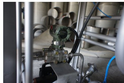
主缸水位压差传感器控制 Pressure transducer for Main level controller
